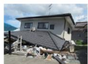
Photo 9-2 Collapse of wooden house after the revision of the Bldg. Standard Law in 2000.
